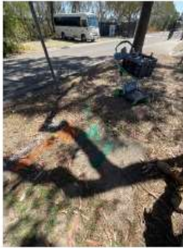
Image 3 – SW32, Stormwater pit cover has no lifting points and cannot be manually lifted by a two-person team.
