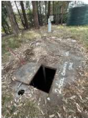
Image 4 – UP04 Large retention chamber cannot be safely investigated without confined space setup.
